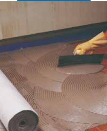
Application of the first layer of Mapelastic, and successive laying of Mapetex Sel
